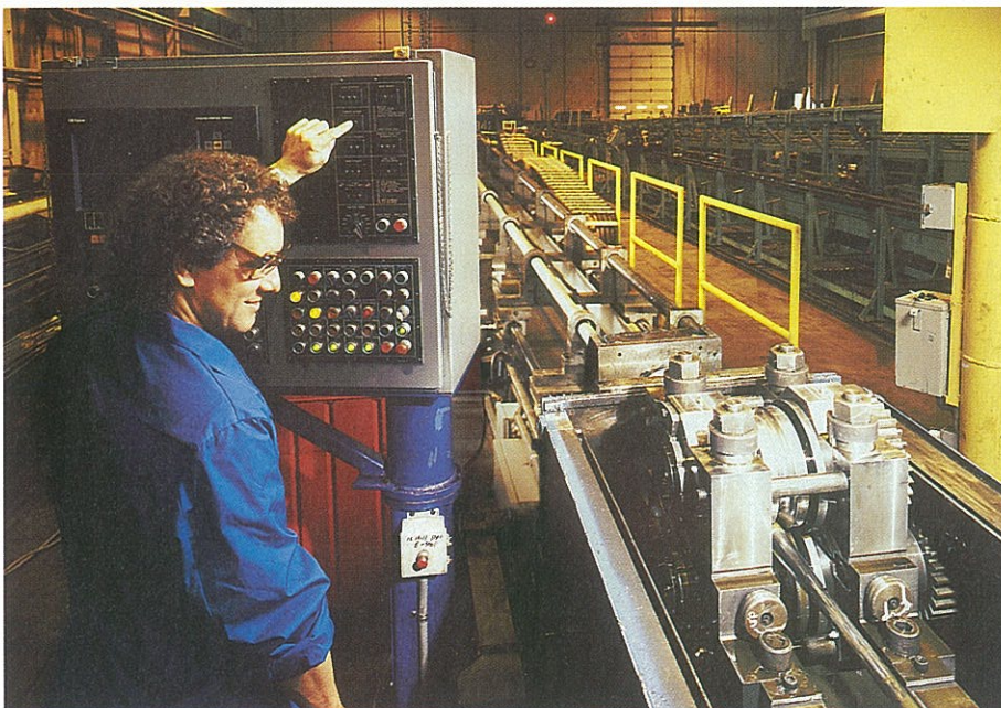
Specially designed pilger mills for the rational production of light-gauge precision tubes have been installed at our facilities in Sweden and the U.S.
